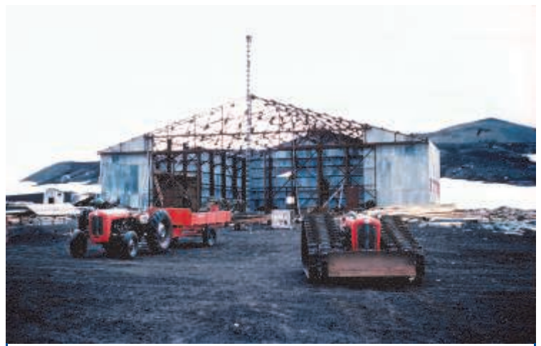
Construction of hangar at Deception Island. AD6/19/3/A30 Photographer: Killingbeck, John Basil (general assistant and Base Leader) British Antarctic Survey Archives Service
