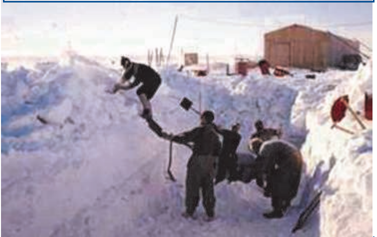
Digging out the generators from the buried generator shed under the snow. The new generator shed is in the back ground. This was the ramp down to the old generator shed with a lid that the Ferguson tractors were driven down to for repairs. Photographer: Bob Lee.
