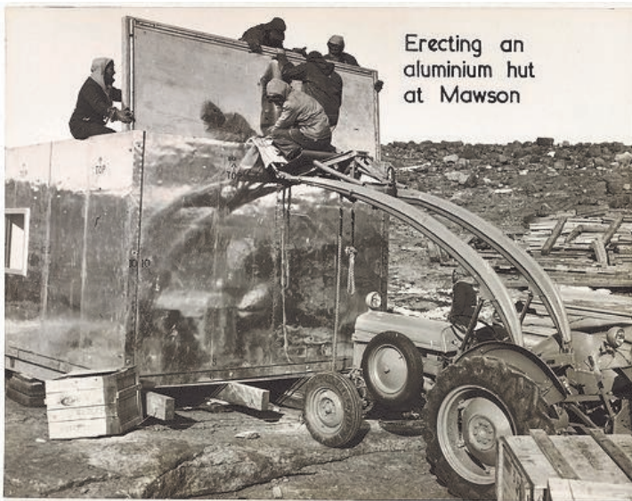
Tractor fork-lift hoists roof onto aluminum hut. Mawson, Antarctica/in Australia in the Antarctic
