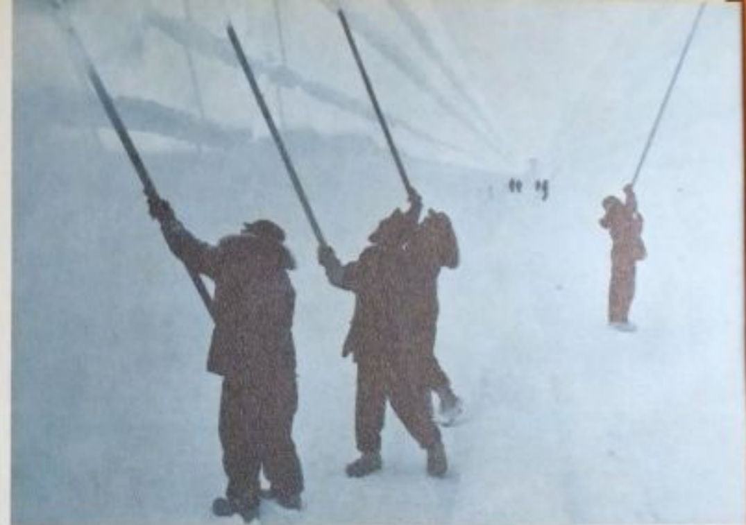
Above: George A. Lewis, BUR 3; Warren W. Brown, BUL3, and Joe L. Crawford, BUL3, scrape loose snow from tunnel walls to keep them smooth.
