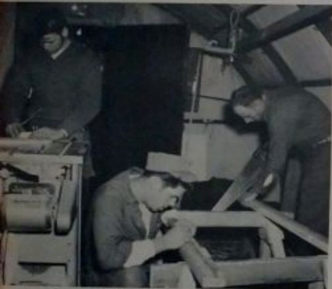
Above: Gary S. Lichtenberger, BUL3; Jerome S. Becmer CN, and Warren E. Brown, BUL3, prepare wall studs for the undersnow buildings at new Byrd.
