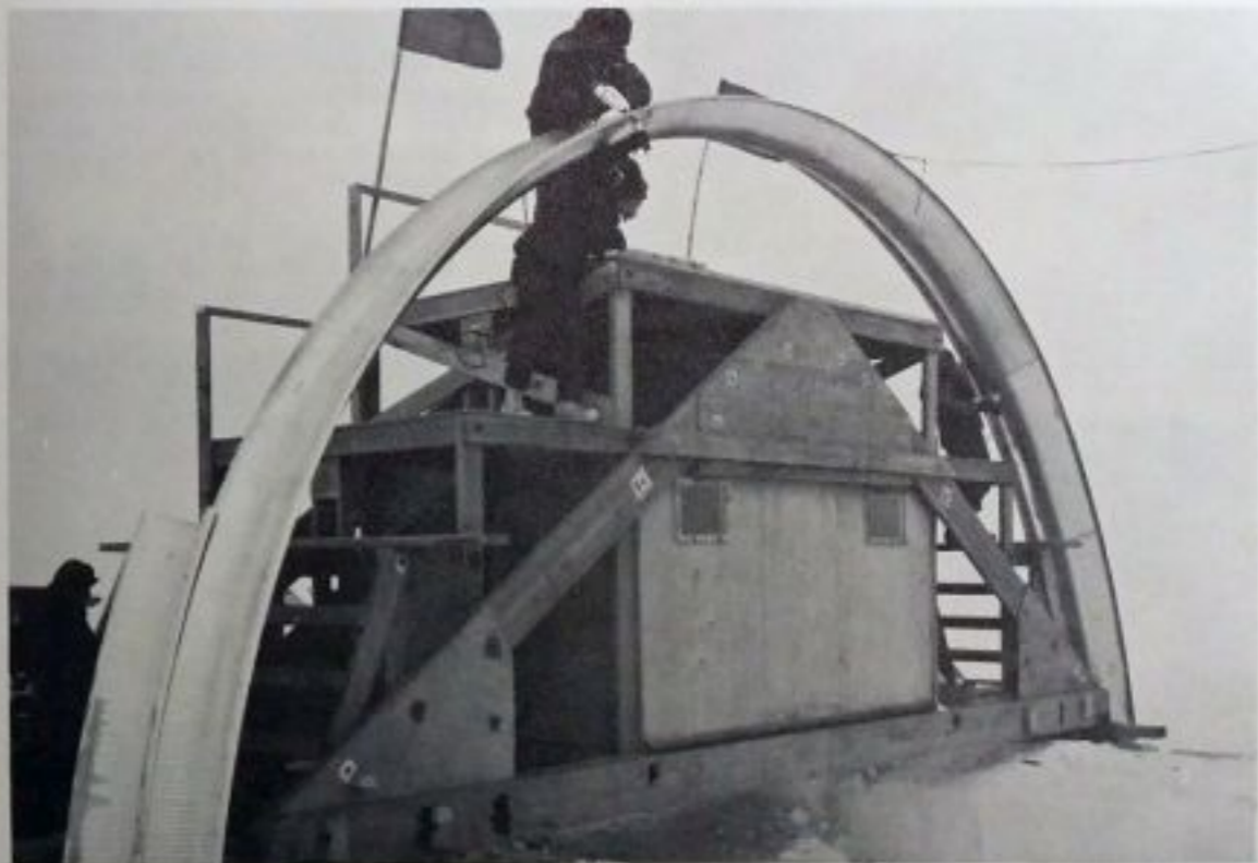
Charles W. Dawkins, CN; Billy L. Talbert, BUL3; Dudley W. Maxfield, BUL3, and Ronald J. Poniewaz, BU2, assemble wondor arch forms which cover the tunnels of new Byrd.
