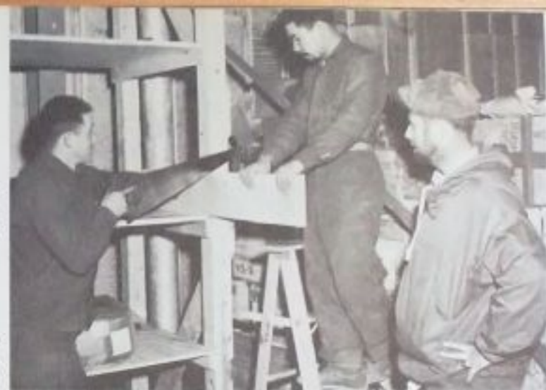
Installing new shelves in supply warehouse, Robert F. Protzman, AKA, saws wood held by Amadeo C. Villianueva, AK2, as Frank Epler, SKC, supervises.
