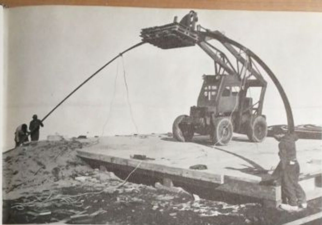
Navy CB steelworkers place a steel arch into place as they construct YX-6's hangar.
