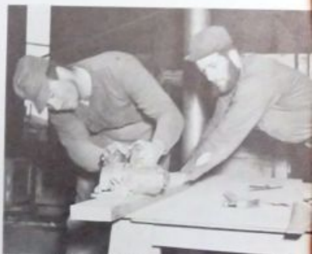
Maynard K. Everett, BUH3, and Lionel W. Morrisette, BULCN, sawing a floor plank to size.
