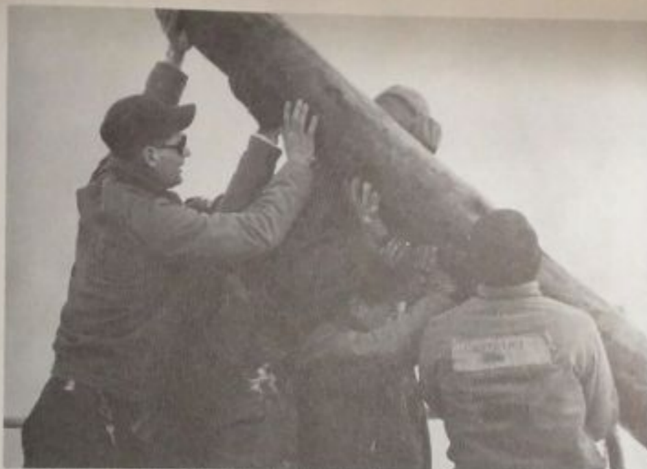
Telephone poles for NAF McMurdo unloaded by Eastwind's crew in McMurdo sound.
